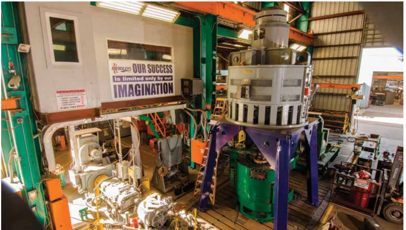
Bradleys, Inc. load tests a large vertical motor on one of its two vertical motor test stands.
